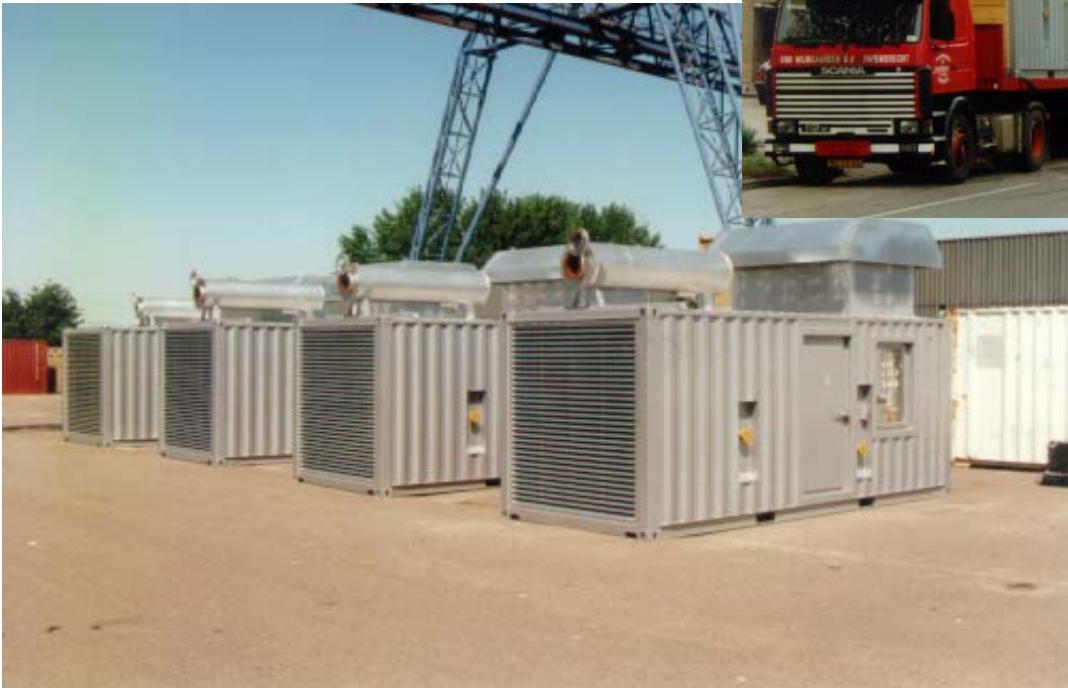
(Above) Transport of the 4 containerized Caterpillar generator sets from Papendrecht to Sri Lanka
