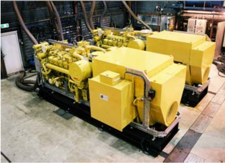
2 Caterpillar 3512B diesel engine driven generator sets
