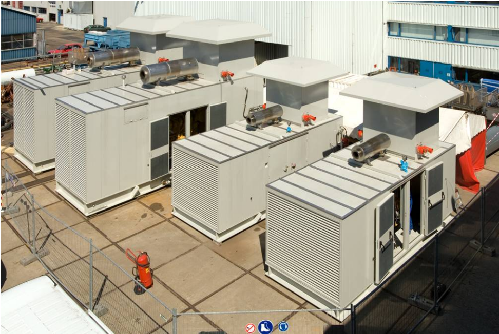
(Above) Gas engine and diesel engine generator enclosure units at FAT test at Pon Power works.
