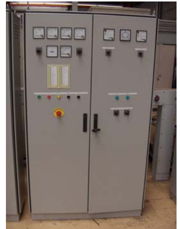
(Above) Unit Control panel
