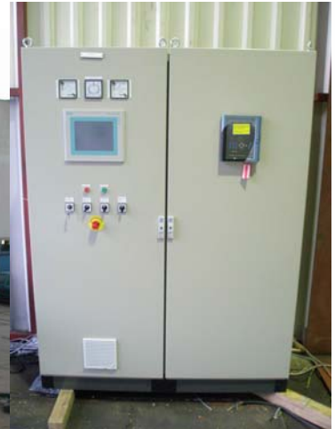
(Above) UCP complete with HMI & Protection Relay
