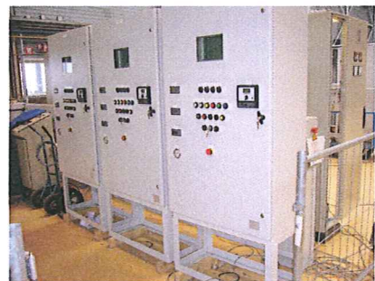
↑ Local Control Panels
