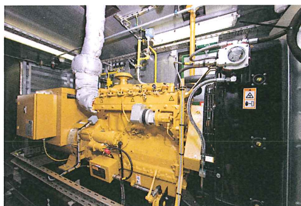
Gas generator package inside container
