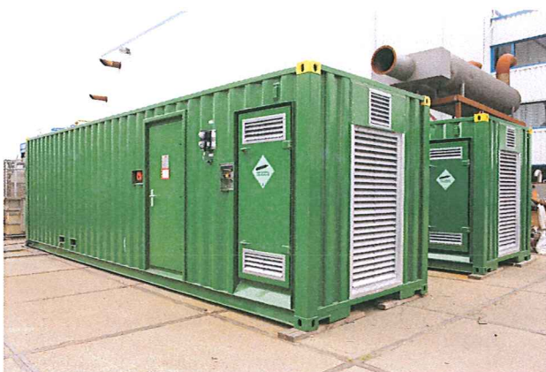
Both Gas units ready for FAT
