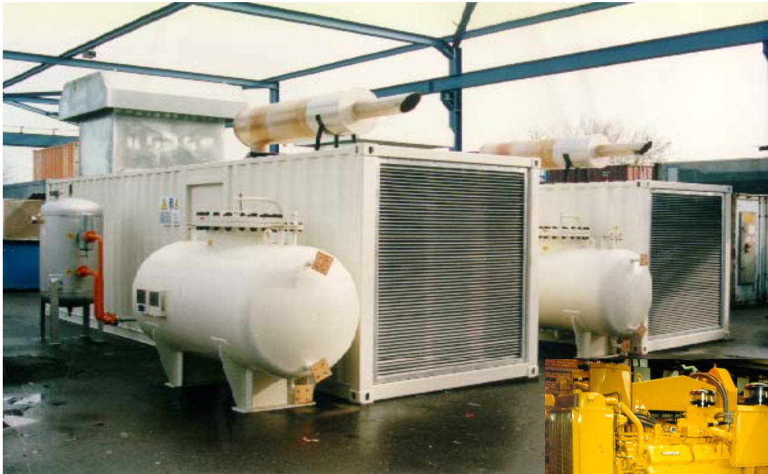
(Left) Containerized genset delivered with fuel tank and air start tank
