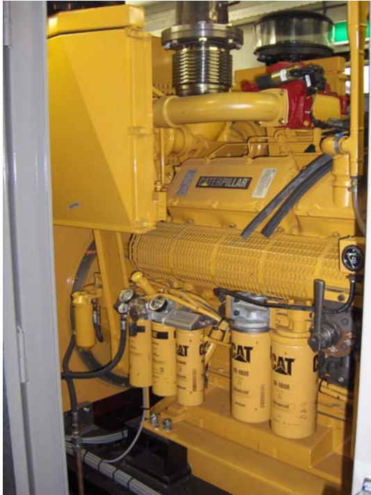
(Above) 3412 Caterpillar engine view inside the enclosure
